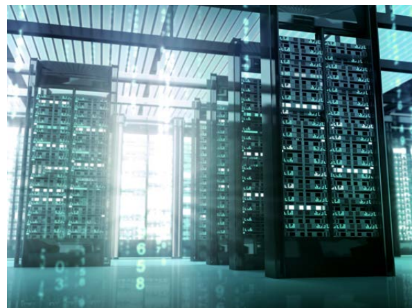
Efficient cooling in datacenters can reduce energy consumption by 30%.
