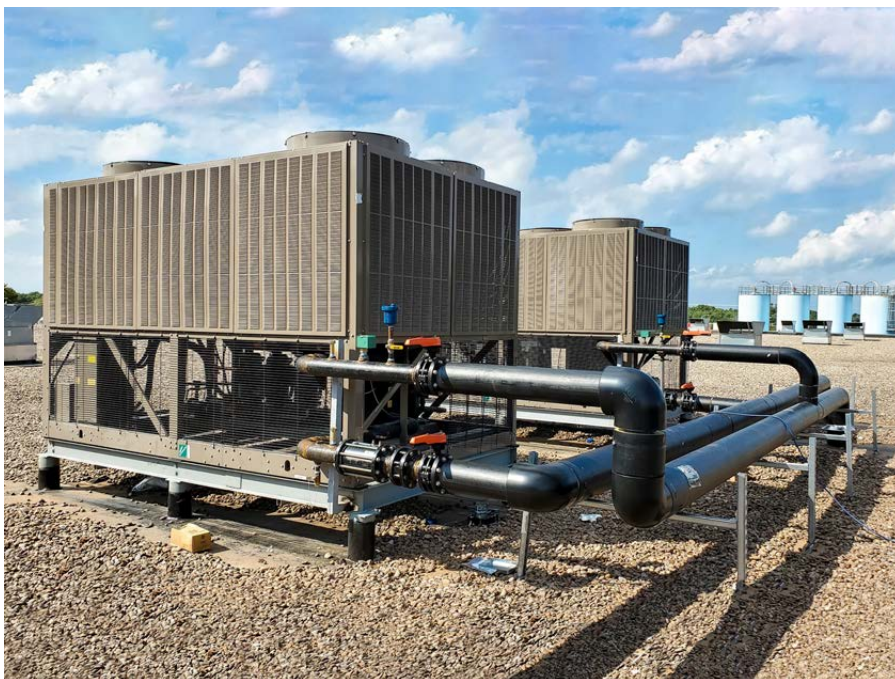
New energy-efficient chiller installation at the plant of GF Piping Systems in Shawnee (USA)
