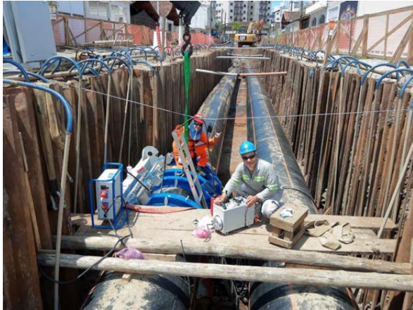
New piping networks in the São Paulo region (Brazil) bring remarkable water savings.
