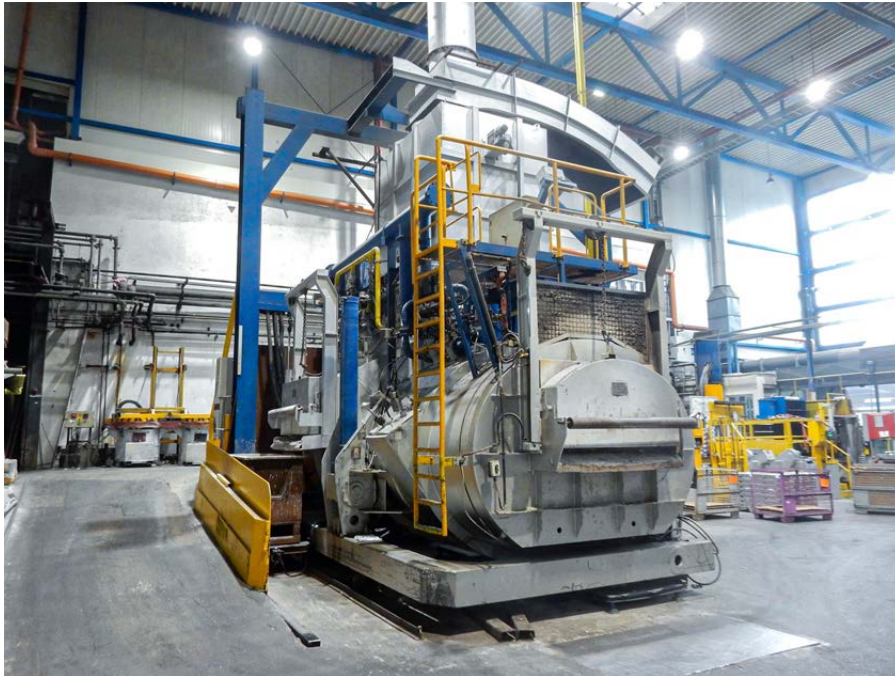
Furnace for aluminum with installed exhaust module at GF Casting Solutions' site in Altenmarkt (Austria)
